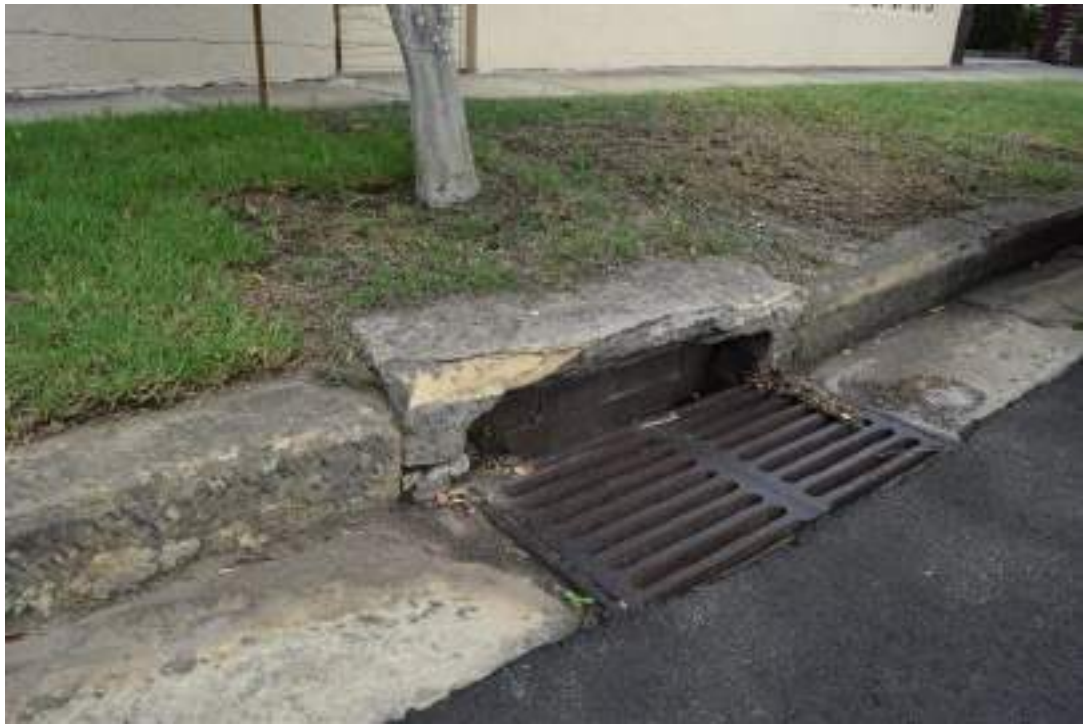
Figure 15: Sandstone kerb, gutters and damaged stormwater drain at 89 Sturt Street.
