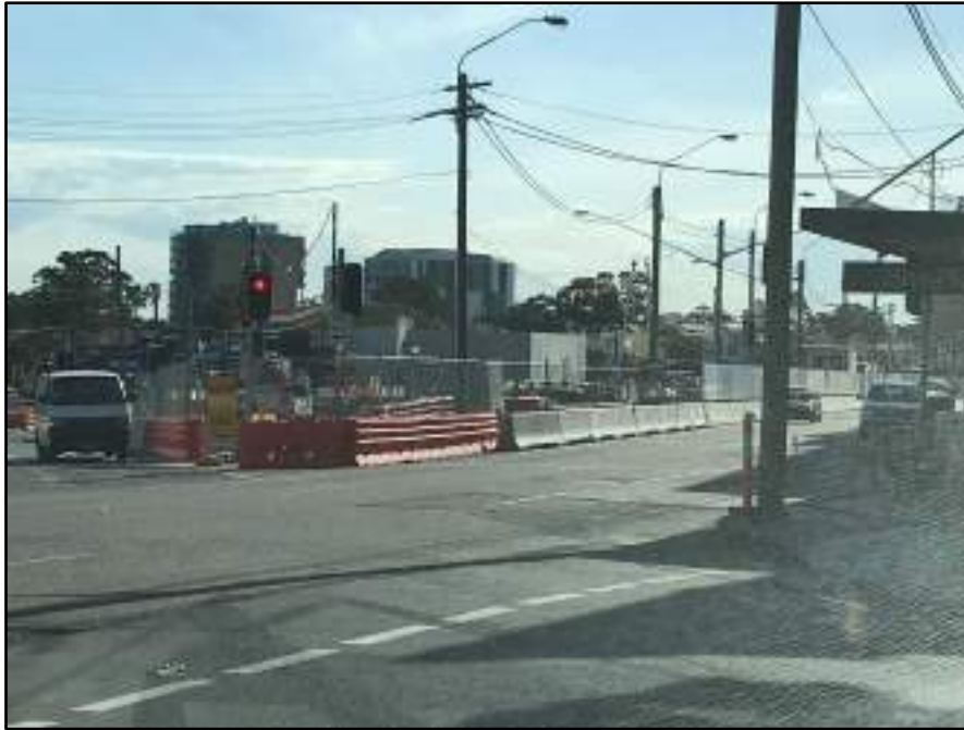
Photograph 9: View of the Kingsford Light Rail Terminus construction site on ANZAC Parade.
