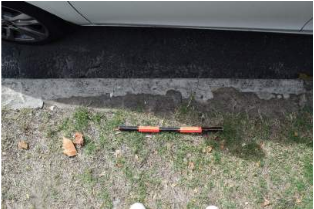
Figure 11: Sandstone kerb with concrete patch repairs at 45 Houston Road.
