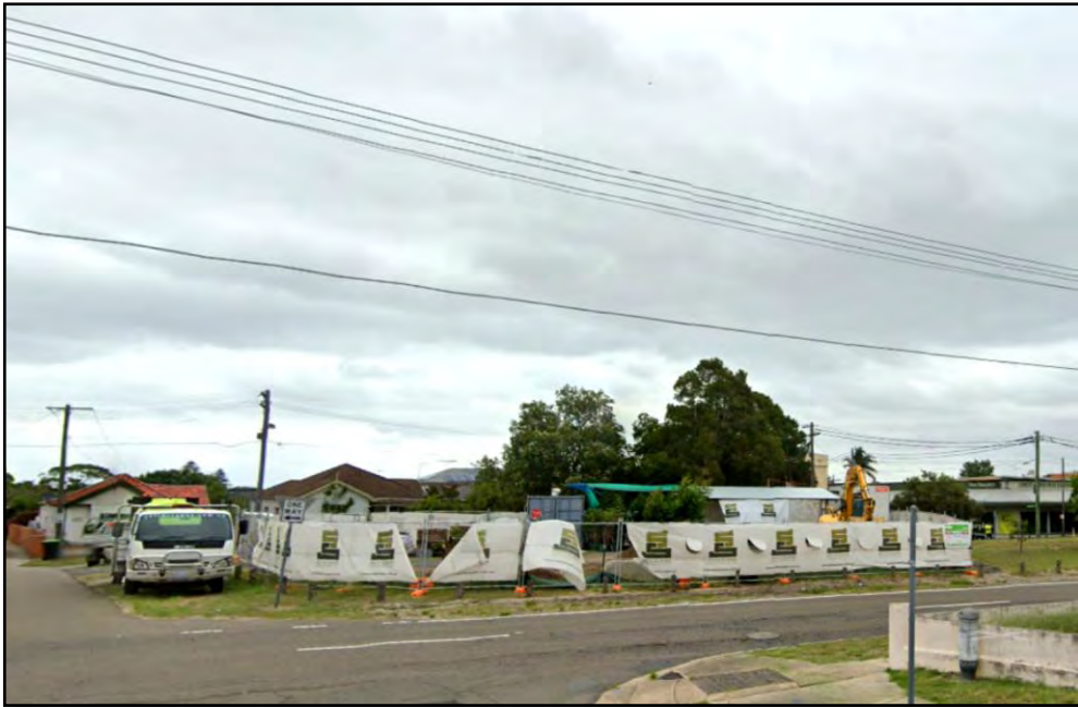
Photograph 3: View of the proposed site for the ANZAC Parade compound on the northern side of Bass Street, currently being used in conjunction with the Sydney Light Rail construction.
