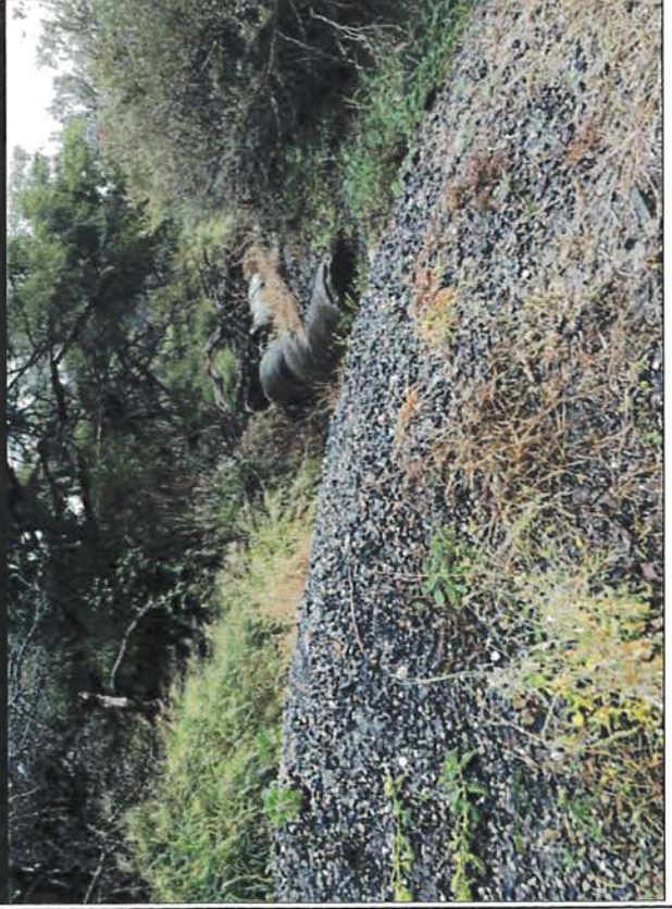
STOCKPILED GRAVELS AND WASTE ADJACENT TO THE ROAD
