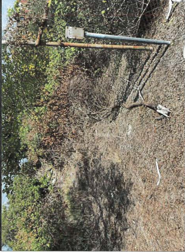
CALTEX PIPELINE INFRASTRUCTURE AND A CLEARED PATH THROUGH VEGETATION RUNNING SOUTH TOWARDS THE BAY
