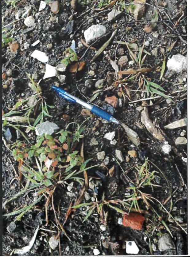
VISIBLE ACM FRAGMENT IN WASTE MATERIAL
