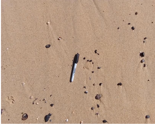
Notes: Visual clearance inspection following removal of suspected asbestos containing FC fragment.
