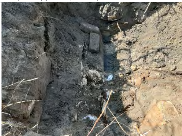
Northern beach, TP03_1.0, Fill with bricks, boulders, minor plastic. Dumped waste up to around 1.5 m.
