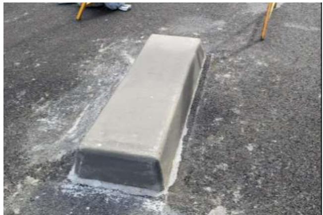
Poured concrete kerb separators for cycleway – Doncaster Avenue, south of Darling St
