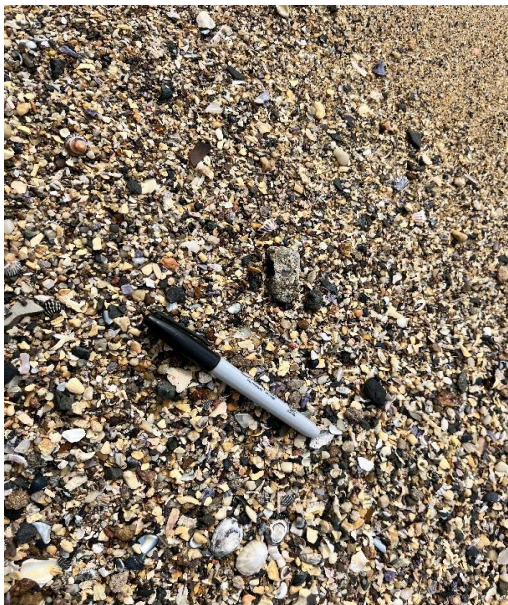
Notes: Visual clearance inspection following removal of asbestos containing FC Sheeting fragment.
